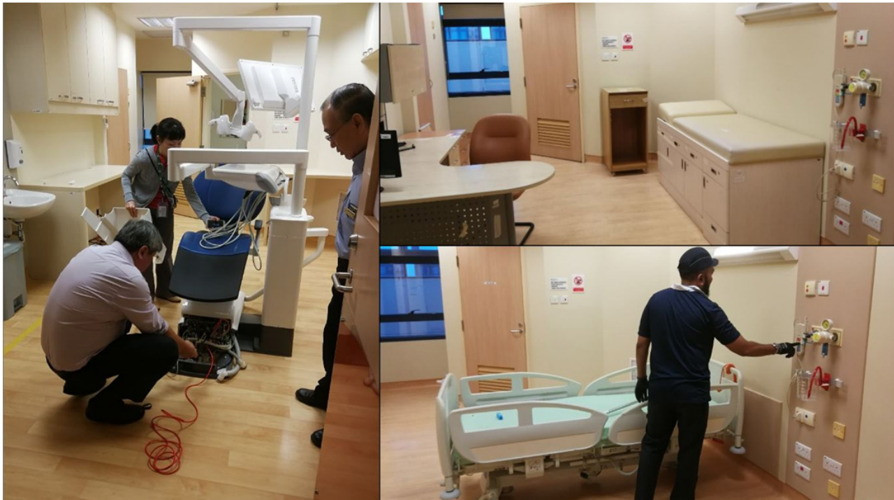
Figure 3. Converting outpatient spaces such as dental clinics and consult rooms into isolation units Clockwise from left: Technicians disconnecting wiring and plumbing prior to shift; An outpatient consult room prior to modification; Performing final tests in modified isolation room.
